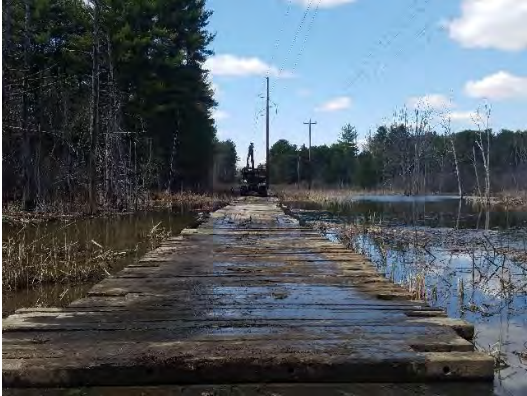
Fig 9: Removing timber mats from access road to Str. 115, through wetland NW11. Viewing northwest. (04-15-20).
