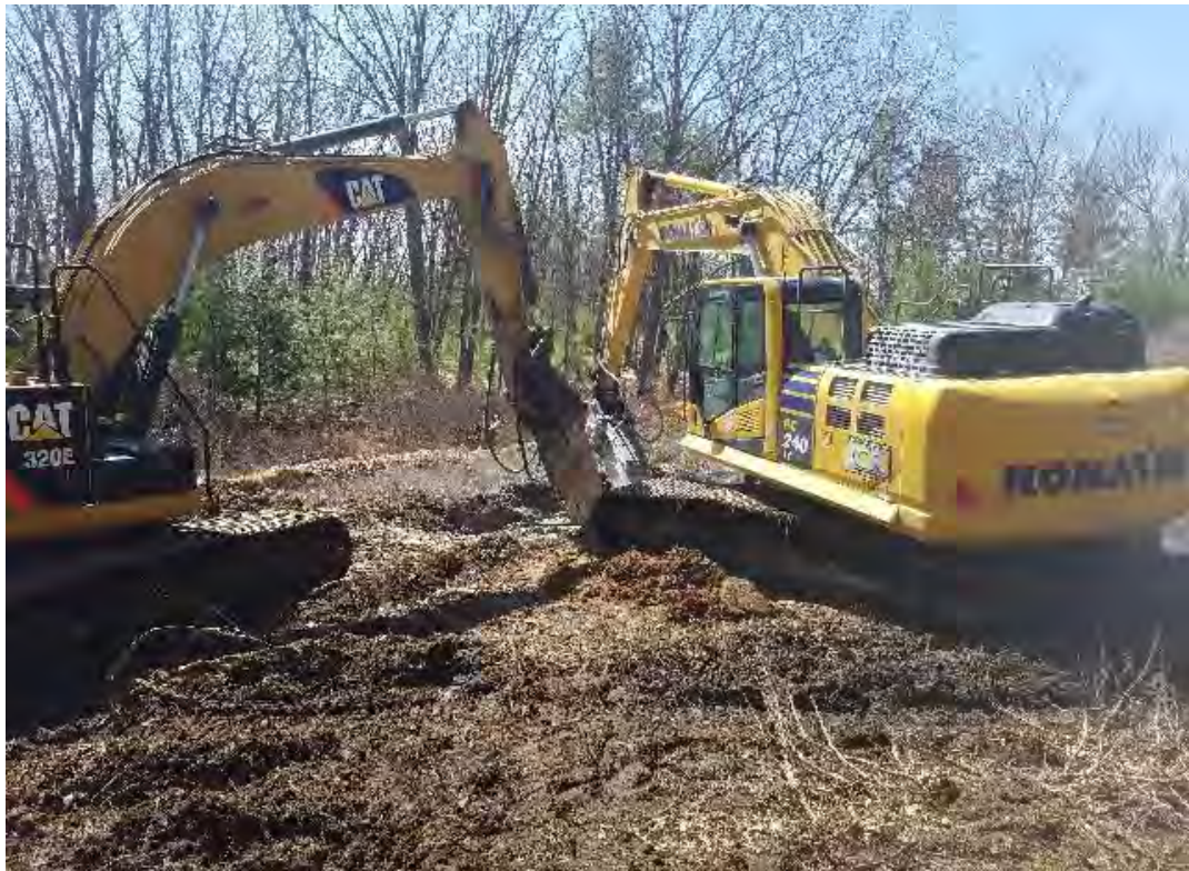
Fig 6: Hammering ledge at Str. 80. Viewing south. (04-14-20).
